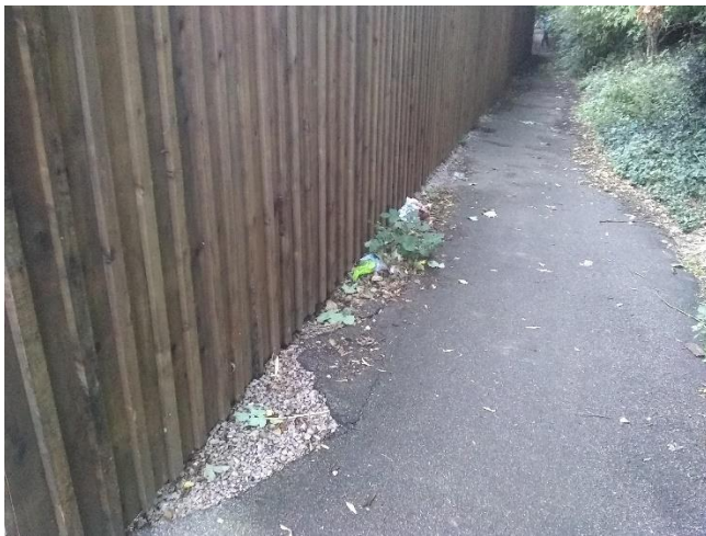
Reduction in width, overgrown vegetation
